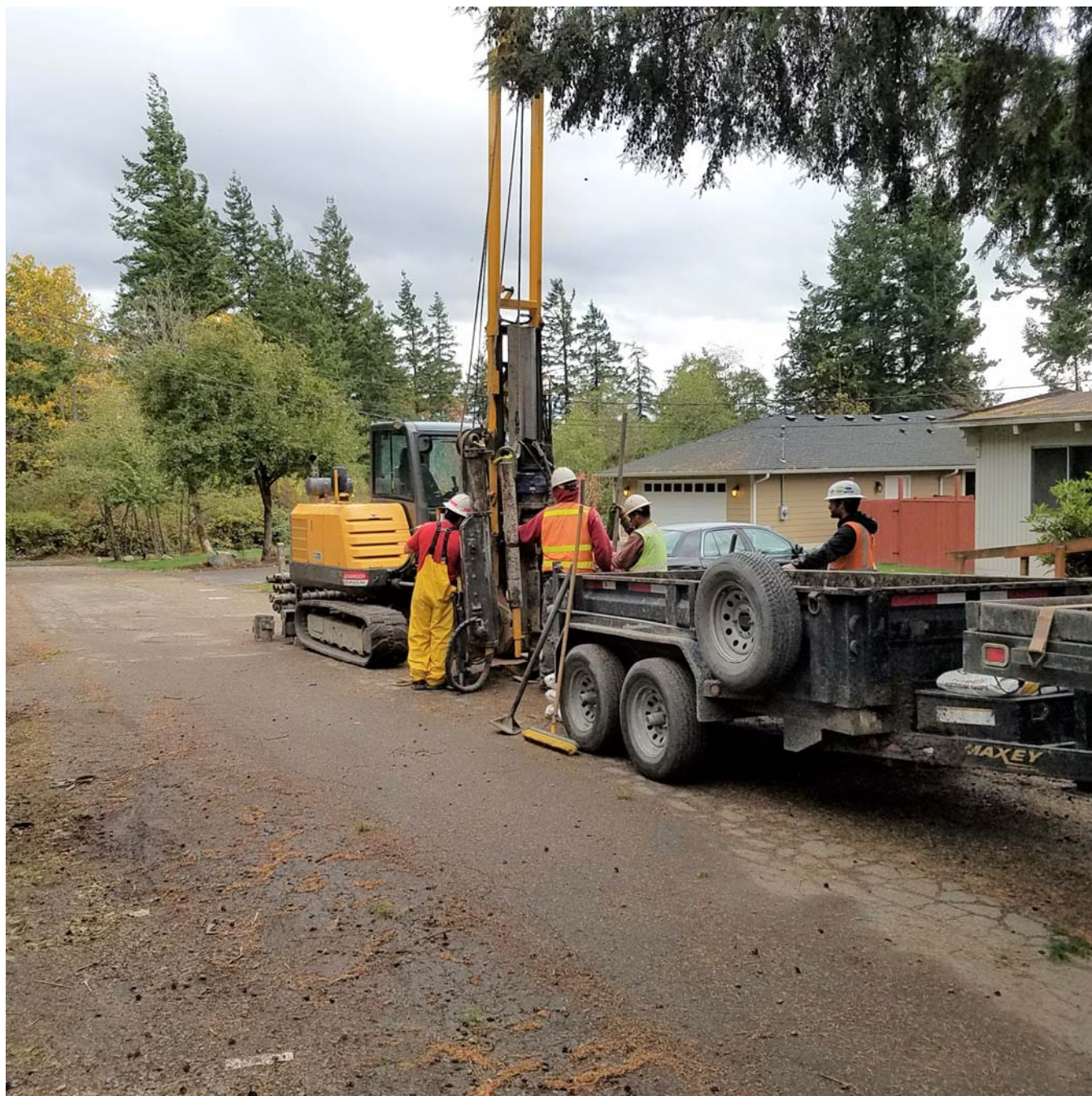
Photo G: Facing southeast on 78 th Place NW near borehole B-2. Photo displays typical cracking along the boundary of the utility corridor under the driller's utility trailer.
