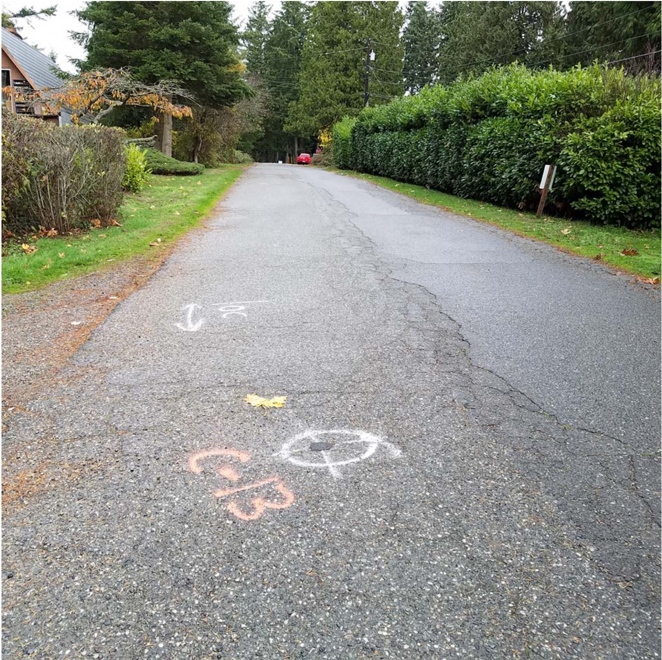
Photo B: Location of core/kDCP C-13 on 42 nd Drive NW. The right of the picture displays a newer asphalt patch over the utility corridor running parallel to the street, and an older section on the left with typical failure due to cracking. The gravel road named 79 th Street NW is in left center of picture. Facing north.
