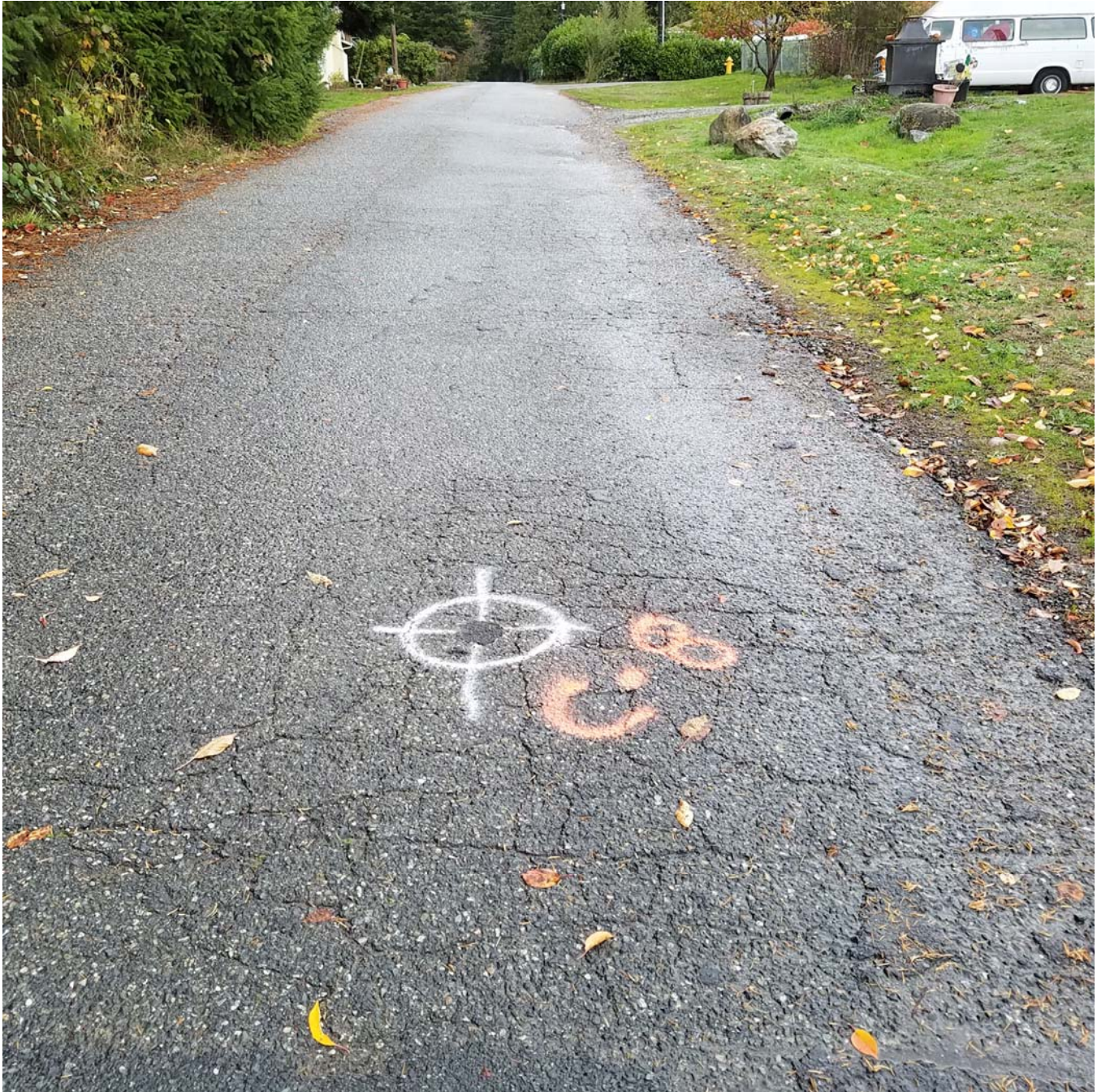
Photo A: Site of core/kDCP C-8 on the south end of 42 nd Drive NW displaying existing conditions. The new pavement edge is at the bottom of the picture, with typical cracking patterns throughout. Facing north.
