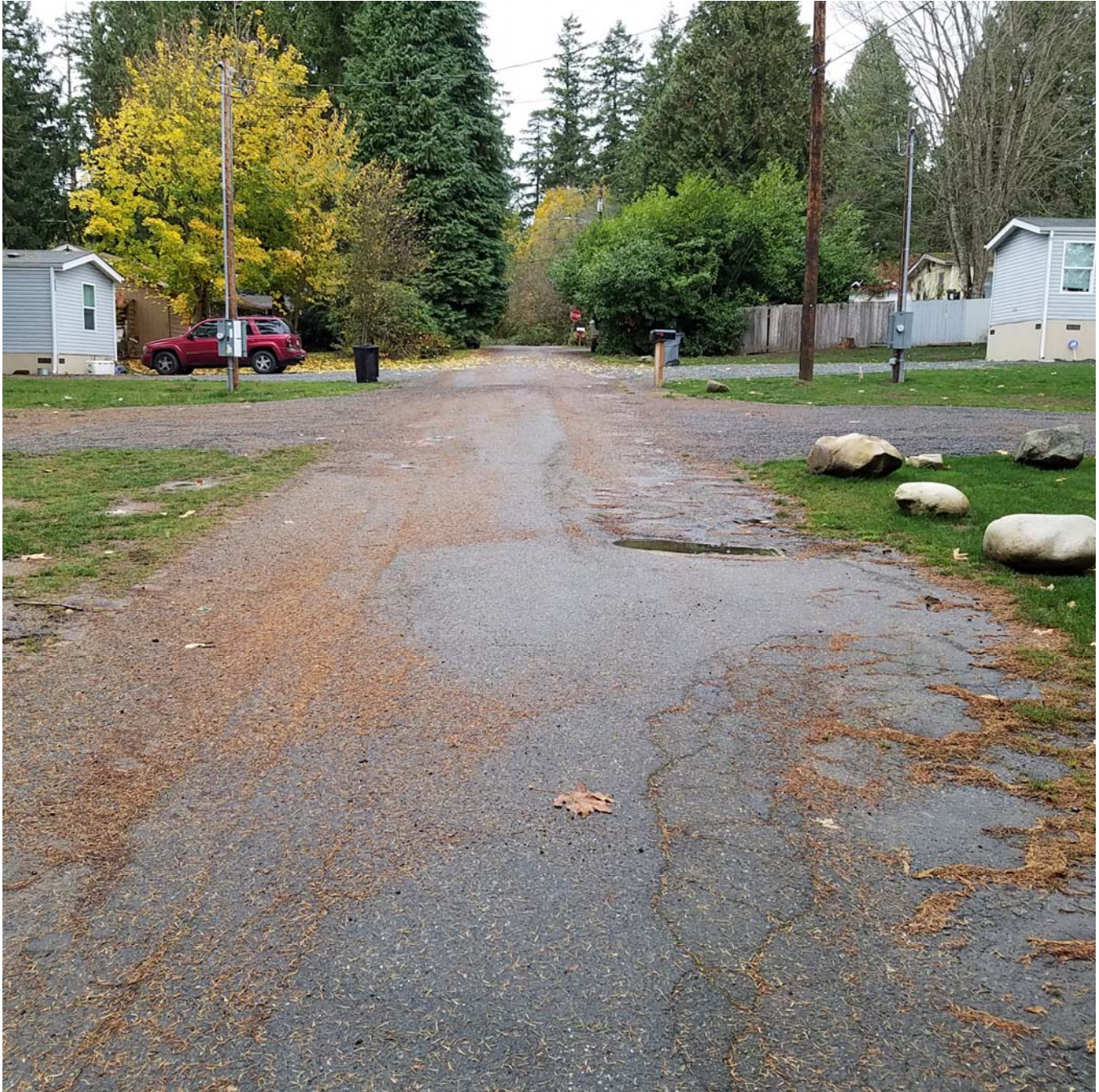
Photo E: Facing west from near the project terminus on 79 th Place NW with stop sign and 42 nd Drive NW in the far distance. Photo displays typical conditions with a utility corridor running the in center of the picture and damaged portions to either side.
