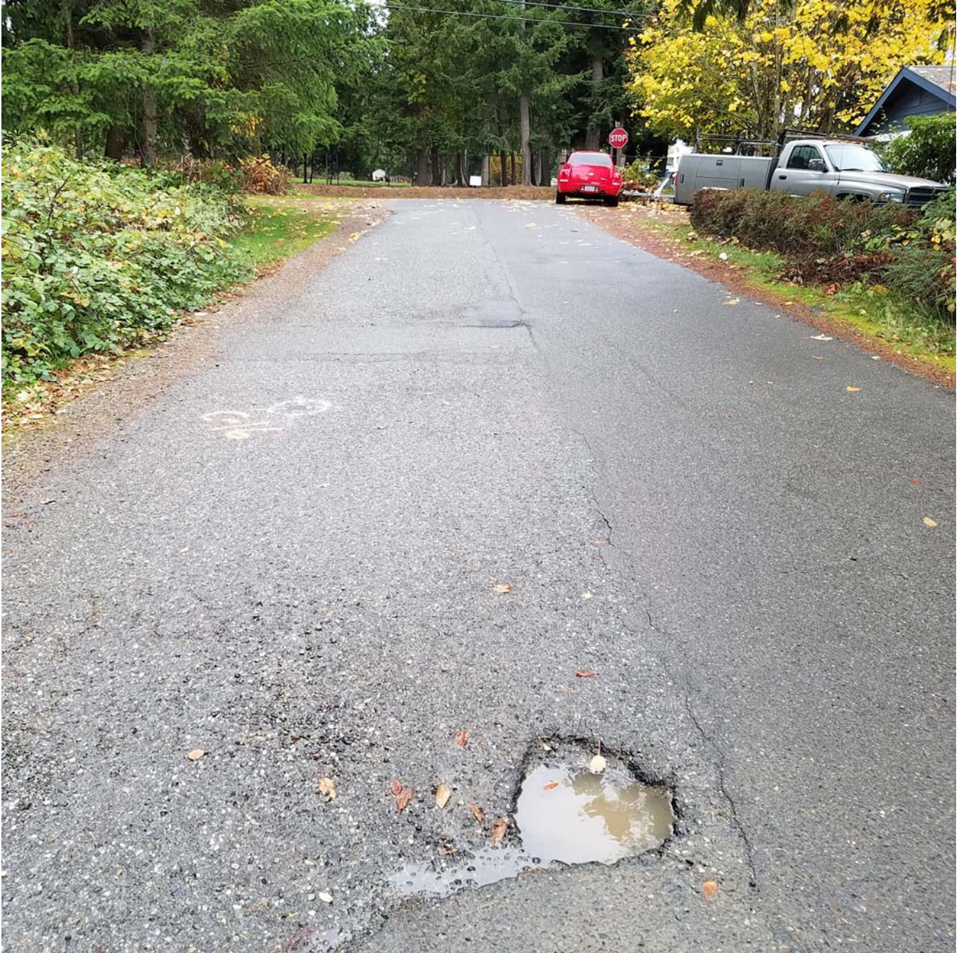
Photo C: Facing north toward Marine Drive near core/kDCP C-16 on 42 nd Drive NW. Photo displays newer utility corridor pavement on the right and older section on the left with damage.
