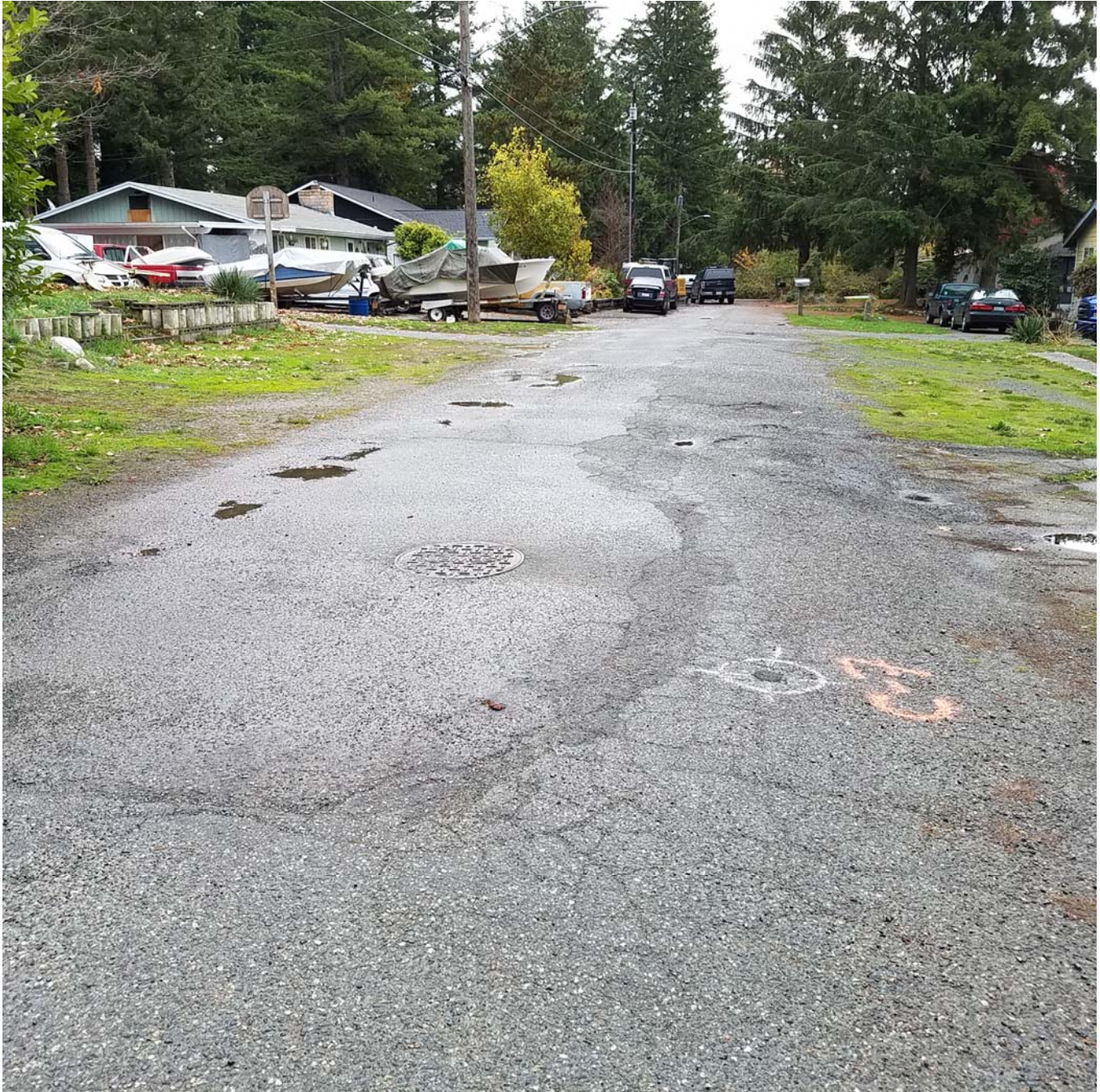
Photo F: Facing west on 78 th Place NW near core/kDCP C-7. Photo displays some of the more significant road damage on the right with a manhole and utility corridor running parallel to the roadway in slightly better condition.
