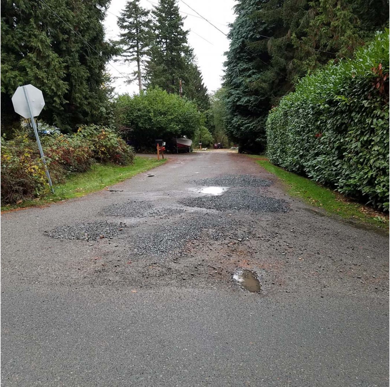
Photo D: Facing east along the alignment of 79 th Place NW with 42 nd Drive NW in the lower portion of the photo. Photo displays heavy damage and temporary gravel patching.
